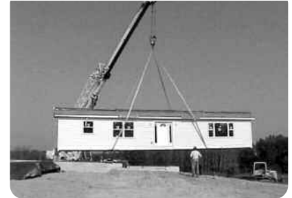
A huge crane lifts the modular home built by students at Washtenaw Community College and sets it on the home's foundation in Milan, MI.
